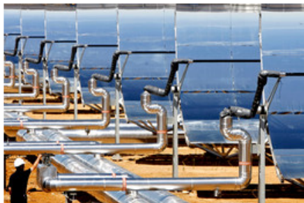
A solar power plant in Alvarado. REUTERS
