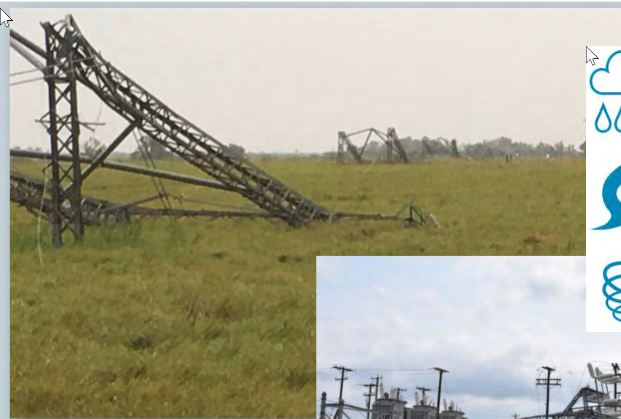
STP-to-Whitepoint 345-kV transmission structures
